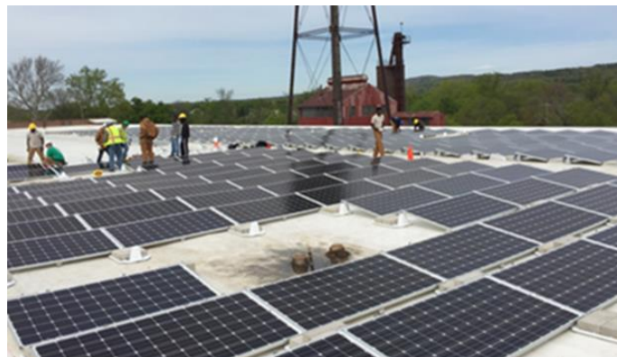
A 144-kilowatt solar array installed by OPRHP staff at Peebles Island, a 190-acre state park located at the confluence of the Mohawk and Hudson Rivers.
