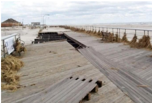
Damage to the boardwalk at Jones Beach State Park from Hurricane Sandy, November 2012.
